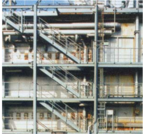
Secondary combustion chamber and boiler
